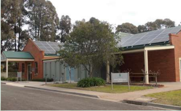
Solar Power Installation
